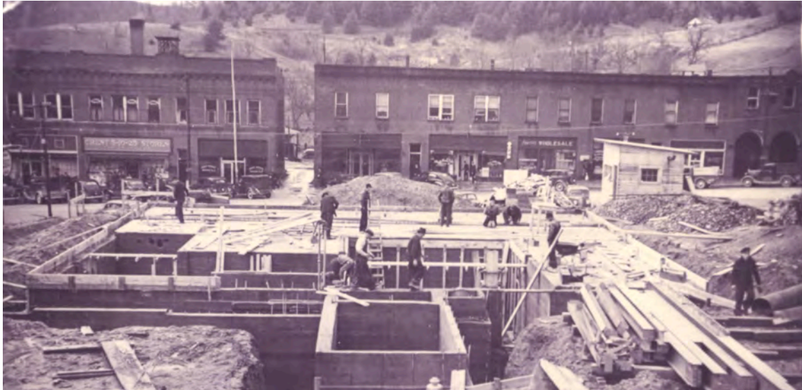
Seen here are workers constructing the US Post Office in 1938. Left to right across King Street are the Farmer's Hardware Block, the Frank A. Linney Block, and part of the Pastime Theatre. Image courtesy of the Historic Boone Collection, Digital Watauga Project.
